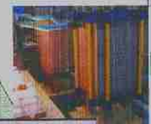
VANADIUM FUEL CELL STORAGE
